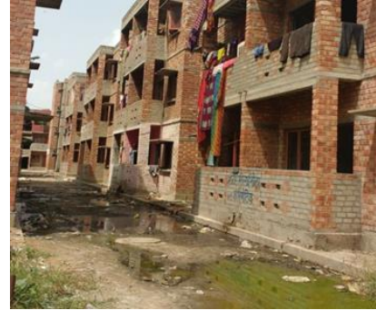
Figure 7: Water logging seen on streets of Bawana housing
